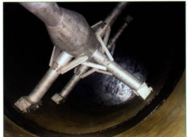
Detail of suction pipes and suction shaft of the FILTROMAX TF filter, flow 10\text{ m}^3/\text{s}
