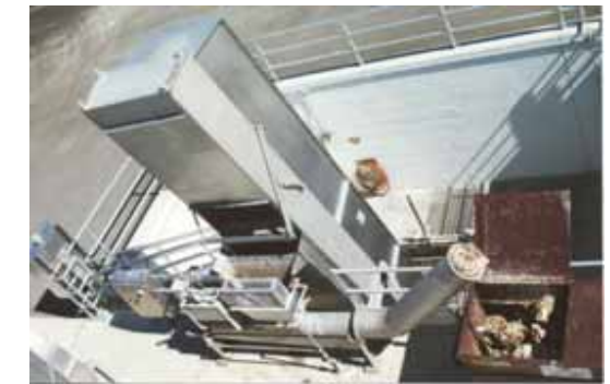
Below: An enclosed Inkos model SRP bar screen discharges screenings into a Inkos horizontal ram press.
